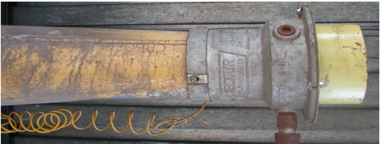
Figure 4 Air Horn Sleeve Connection
